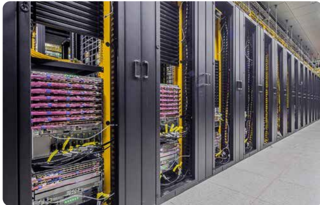
Data center server rooms are equipped with dual redundant power supplies via overhead trays, to ensure reliable service operation
